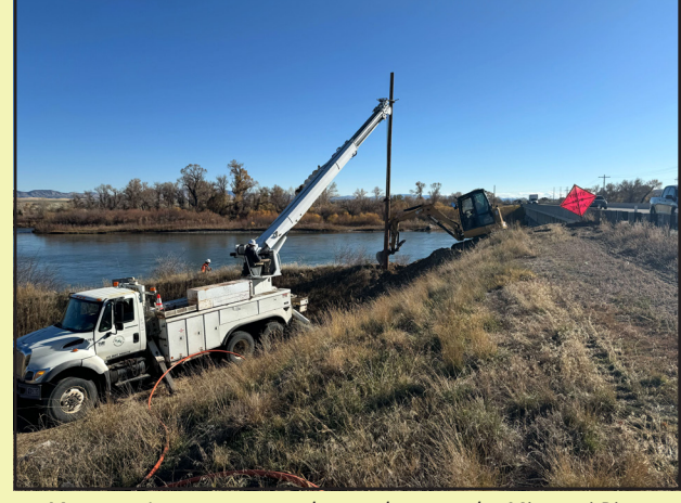
Montana Internet crews place poles over the Missouri River leading into Townsend which will connect fiber cable from Townsend Elementary School to Spokane Creek Road. Photo Provided by Montana Internet
