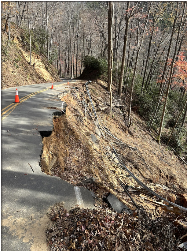
Road washout on NC State Highway 80 north of Marion, NC. Photo Provided by Philip Knaub
