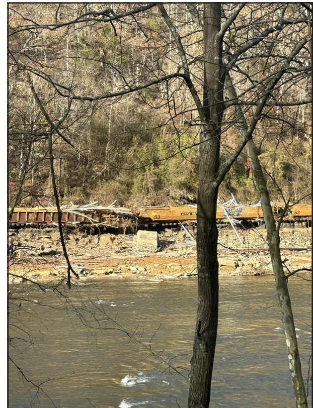
Washed out train tracks and rail cars covered with PVC pipe that was washed downstream in the Swannanoa River. Photo Provided by Philip Knaub
