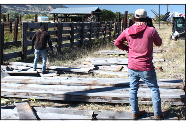
Two crew members from Onsite Management contractor Kendall Carpenter stack weathered planks at the Livestock yards. Nancy Marks, MT43News Photographer
