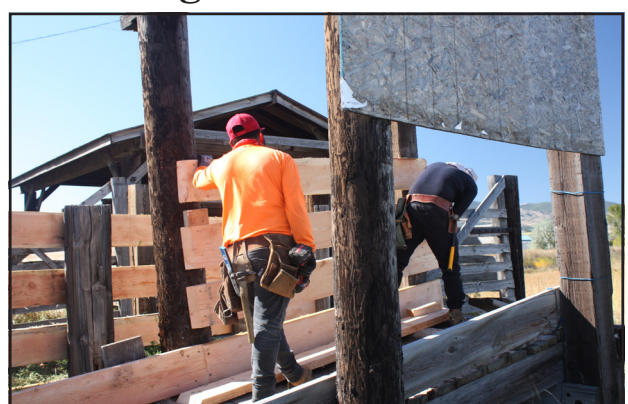
Loading ramp at Townsend Livestock Yards is rebuilt. Nancy Marks, MT43News Photographer
