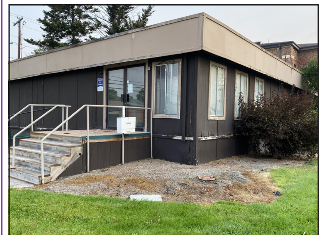
The former Family Medical Clinic building is in need of major repairs to the roof, siding, skirting, and HVAC and will be sold to the highest bidder willing to remove the building from county property. Photo by Linda Kent
