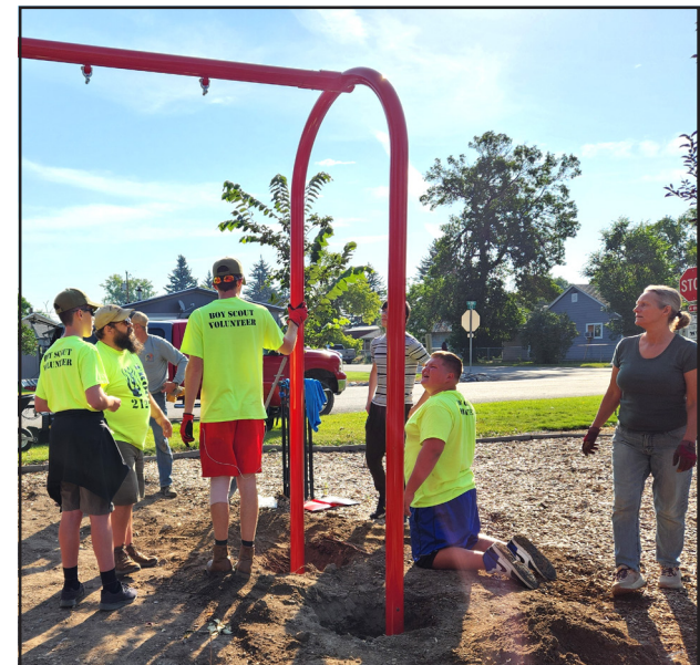
Lots of work, digging holes and setting level swing sets. Damon, Eric Sommer, Walker Young and Aiden Mosher (kneeling). Photo Credits: Dee Gannon
