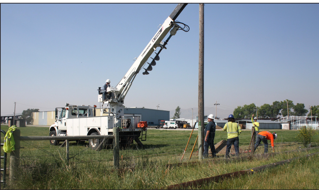
Lineman apprentices learn to operate the Digger Derek used to set electrical poles. Nancy Marks, MT43News Photographer
