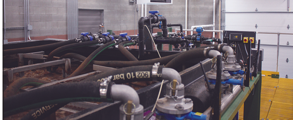
Tanks in Wastewater Treatment Plant Photo Credits: Nancy Marks
