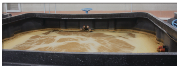
Sludge moves from the outside holding unit to a small building which houses four holding tanks. Sludge is oxygenated, then moved through anaerobic processes which break down the waste. Photo Credits: Nancy Marks
