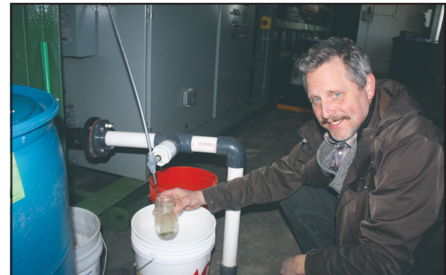
Sigler displays the almost clear, nonpotable water as the final product of the MBR system. Photo Credits: Nancy Marks
