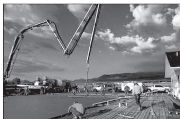
Bill Lane Construction workers put the finishing touches on the concrete slab for Trailhead church's expansion July 11. Photo Credits: Chuck Blair
