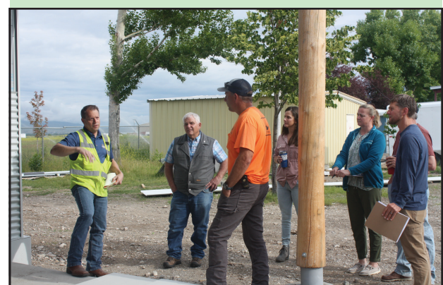
Architect Scott Cromwell, Slate Architecture, explains the progress on improvement work at the Fairgrounds 4-H Building June 27. Left to right: Cromwell; Commissioner Darrel Folkvord, AV Contractor Mike Albrecht; Commissioner Lindsey Richtmyer; Fair Manager Jessica Erickson; Fairgrounds manager Bill Malone(behind) and Great Western Engineer Karl Yakowick. Photo Credits: Nancy Marks
