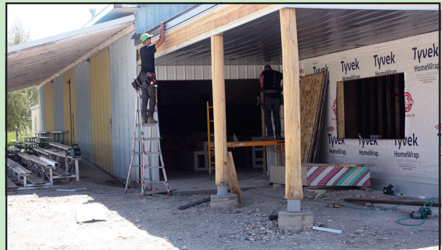
Dick Anderson Construction workers shown attaching roof for the Fairgrounds Livestock Pavilion last week. Photo Credit: Nancy Marks
