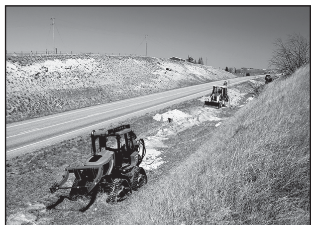
Blackfoot Communications of Missoula's crews installing fiber optic cable along Highway 12 East for Townsend small businesses. Photo Credits: Nancy Marks
