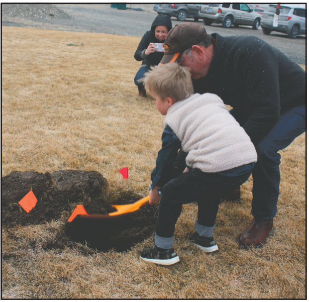
Waylon Nix age four, of Winston digs the first hole for the building expansion at Trailhead Church with help from Expansion Committee member Chuck Blair.
